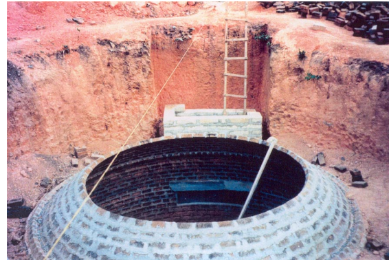
Fig. 9: Biolatrine for 2x3 toilets, 200 people in Kumasi, Ghana (under constr.) front: digester, rear: influent shaft (Source: [3])
